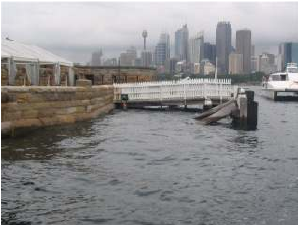
Figure F2: Western Seawall at 0915 hrs. Measured water level is 1.95m ISLW (1.025m AHD).
