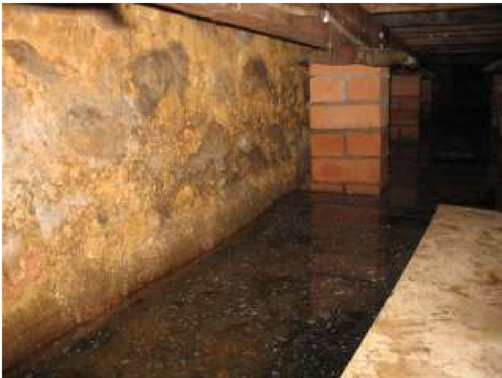
Figure F12: Ocean ingress beneath sub-flooring of function room in the Barracks at 0945 hrs. Measured water level is 1.90m ISLW (0.975m AHD).
