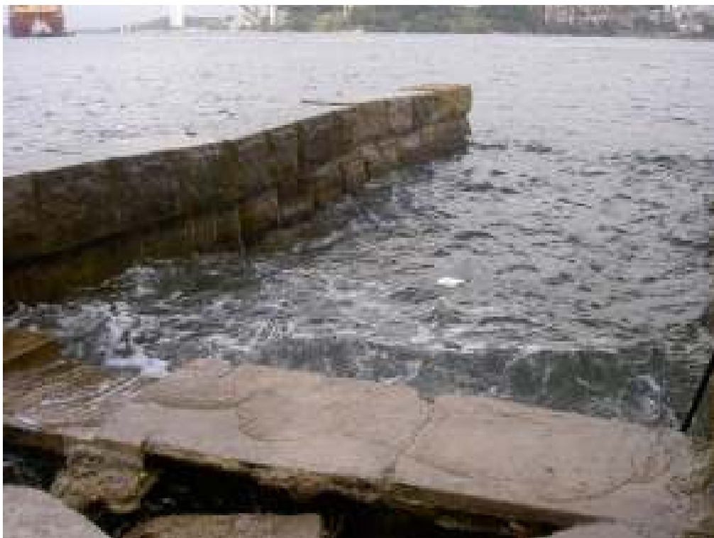
Figure F6: Slipway at SW end of Fort at 0845 hrs. Measured water level is 1.95m ISLW (1.025m AHD).
