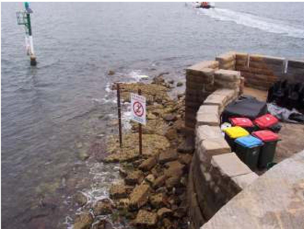
Figure E2: Rock berm apron at base of south-western seawall exposed at low tide.
