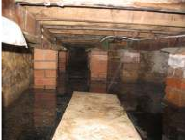
Figure 8.1: Existing seawater ingress below flooring system (approx 1.90m ISLW)
