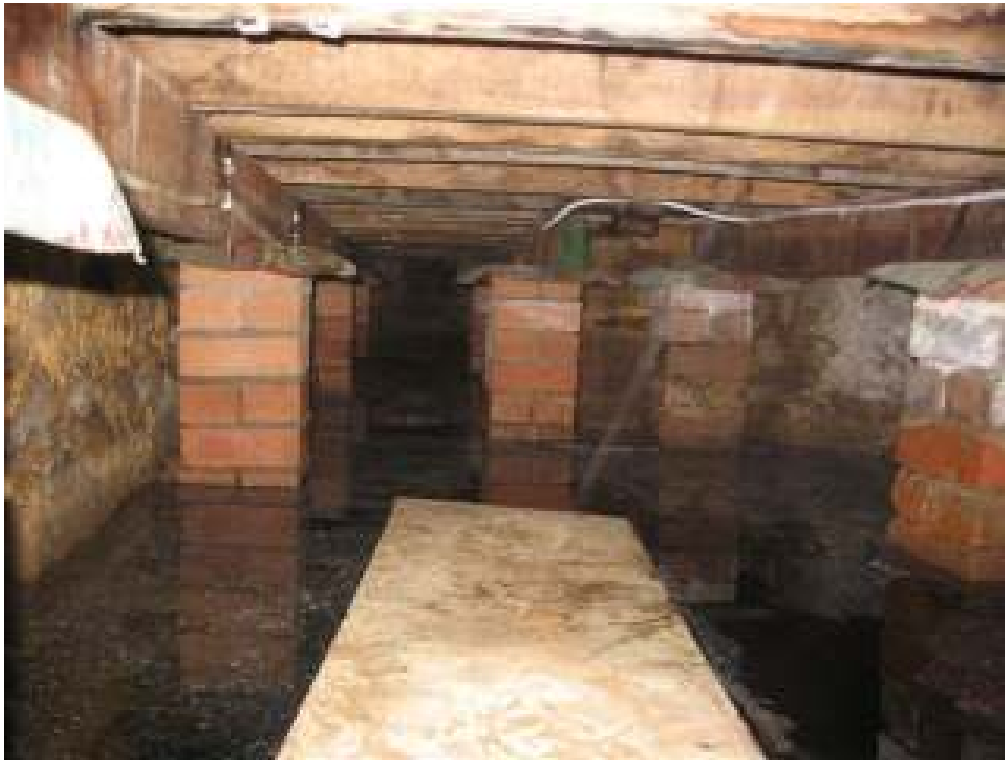
Figure F11: Ocean ingress beneath sub-flooring of function room in the Barracks at 0945 hrs. Measured water level is 1.90m ISLW (0.975m AHD).
