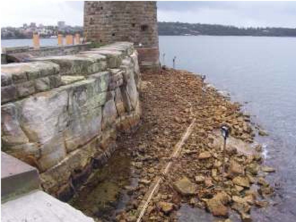
Figure E1: Rock berm apron at base of eastern seawall exposed at low tide.
