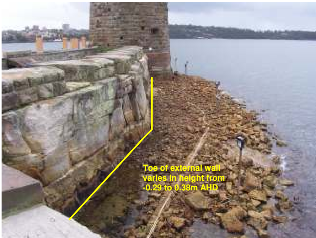
Figure G7: Eastern Seawall and Martello Tower exposed at 1145 hrs (low tide) on 6 November 2007. Measured water level is 0.48m ISLW (-0.445m AHD).
