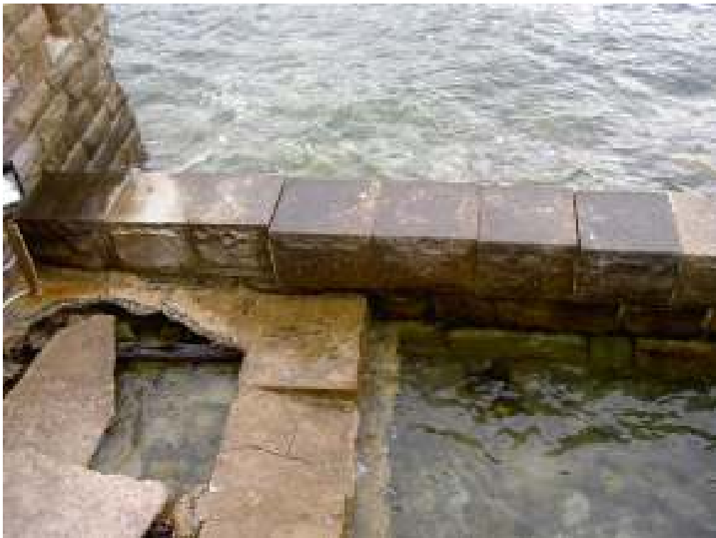
Figure F8: Slipway at NW side of Fort at 0915 hrs. Measured water level is 1.95m ISLW (1.025m AHD).
